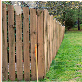
This fence encroaches onto a neighbor's property
