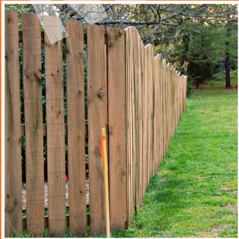
This fence encroaches onto a neighbor's property
